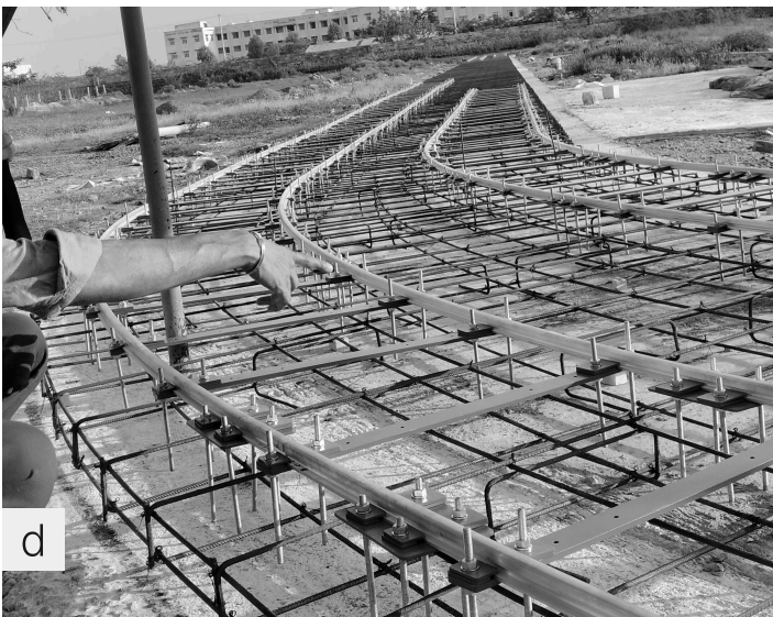
Stages of the site preparation at Karapakkam, Chennai captured from November 2025 to early March 2026.
